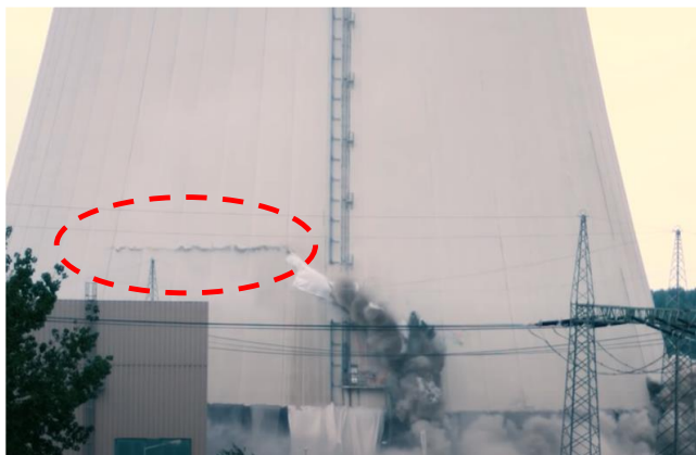
Figure 9: Cracking in the tower shell immediately after the ignition of the explosive charges
